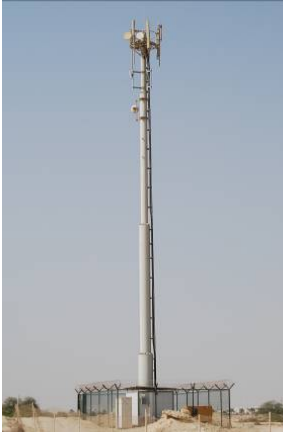
Normal Mobile Base Station
